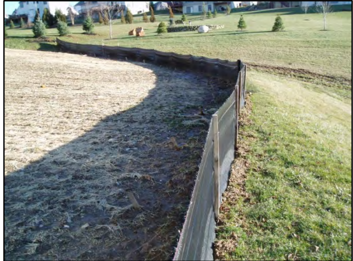
Figure 157. Silt fence (York County Conservation District 2009).
